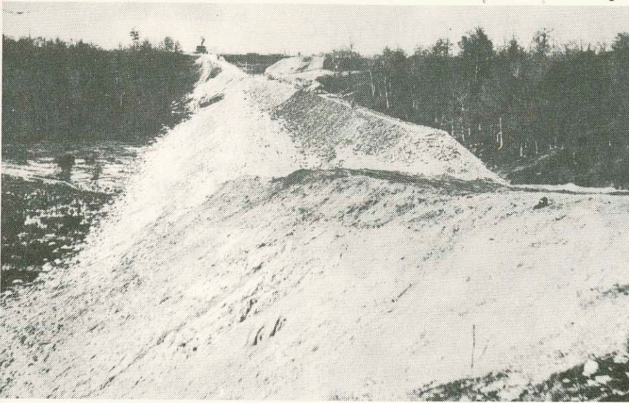
The big cut and fill going into Manitowoc on the Wisconsin Central. The fill area in the center of the photo is just North of Lindbergh Drive.
